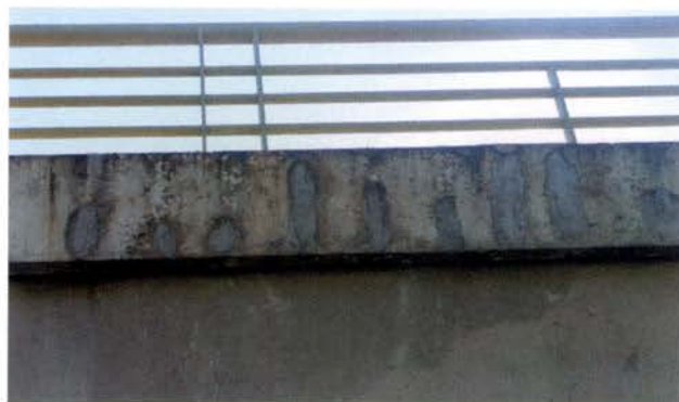
Figure 37. Fissuration des ragréages
